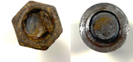
Fatica + corrosione / stress corrosion
